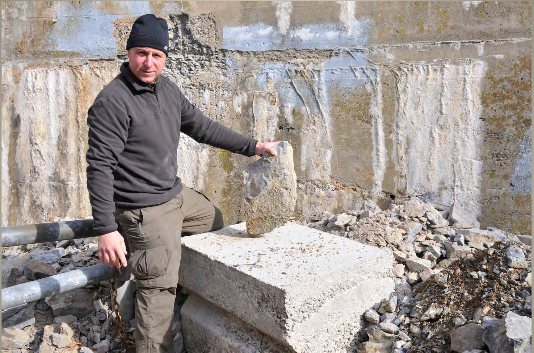
Contractor Steve Ferrari holds typical spalled stone removed from tunnel ceiling
