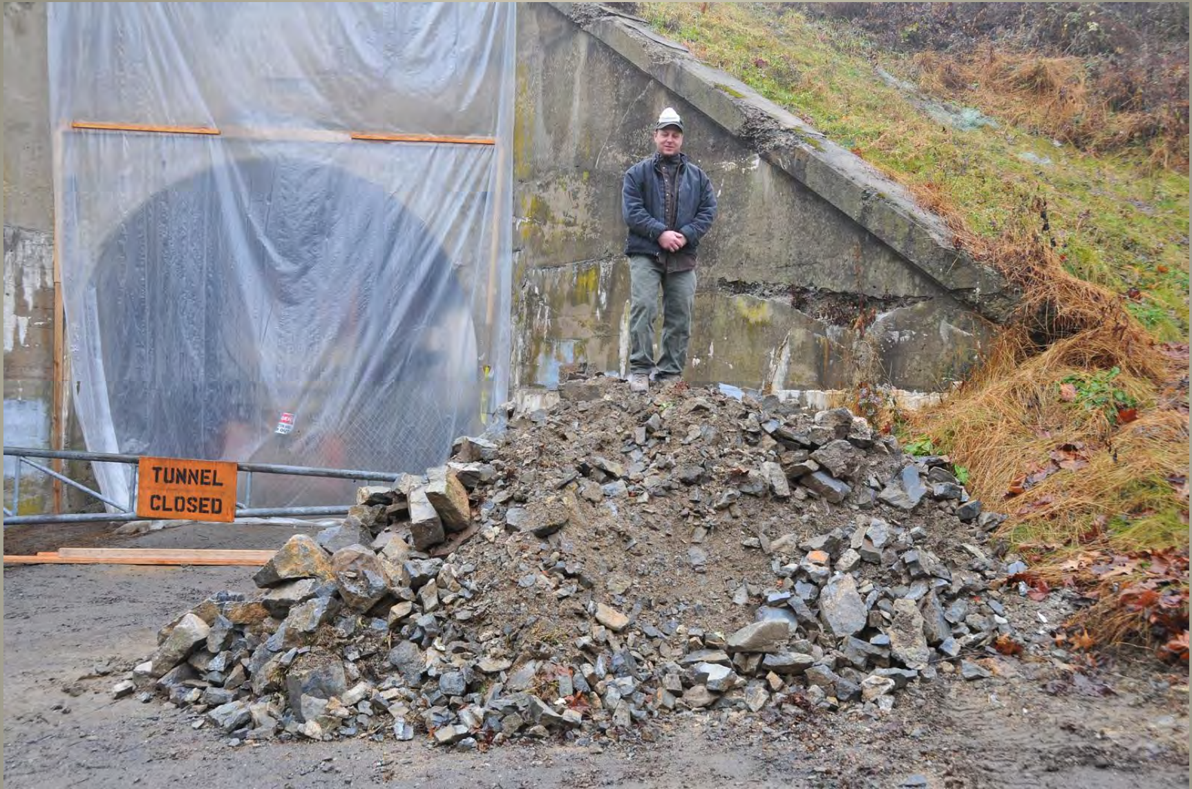
Some of the spalled and fractured stone removed from the surface of the tunnel.
