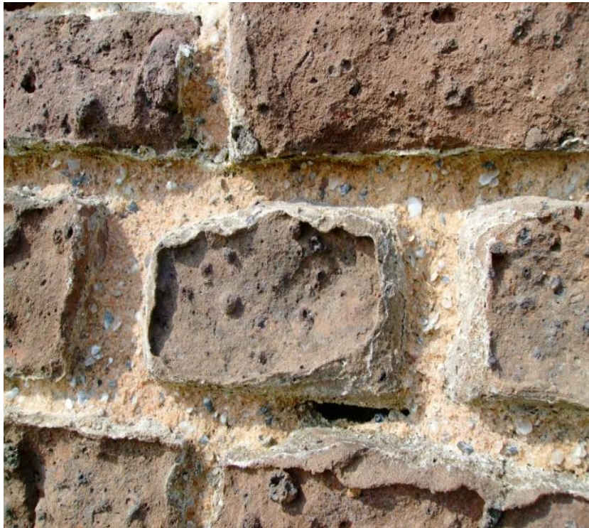
Original Rosendale-Lime-Sand Mortar after Wearing Away of Portland Pointing Mortar Installed In the 1960's
